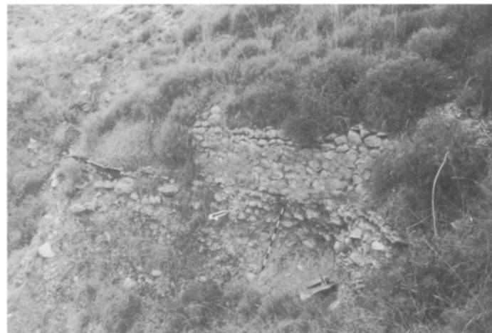
d. Anaploga River: remaining side wall of channel after collapse into ravine, from east
